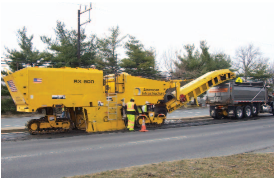
On March 4, Maryland awarded a $2.1-million road resurfacing and improvement project along New Hampshire Avenue in Montgomery County to American Infrastructure. (Photo courtesy American Infrastructure)
